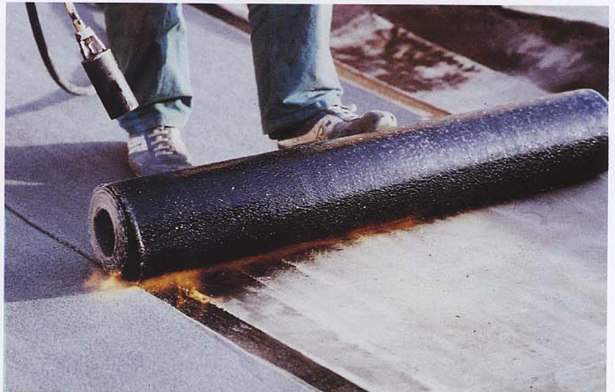
Torch-on application of the membrane. Detail showing the correct position of the roll and the colour of the flame.
